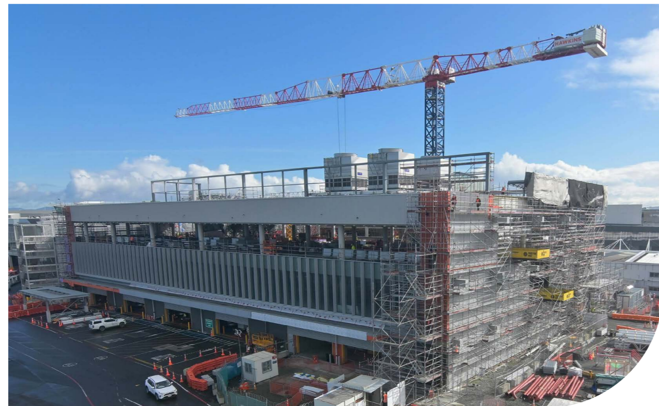
2 Windows being installed on 'the Stitch' in August 2024. The structure will provide a seamless link between international and domestic jet travel.
