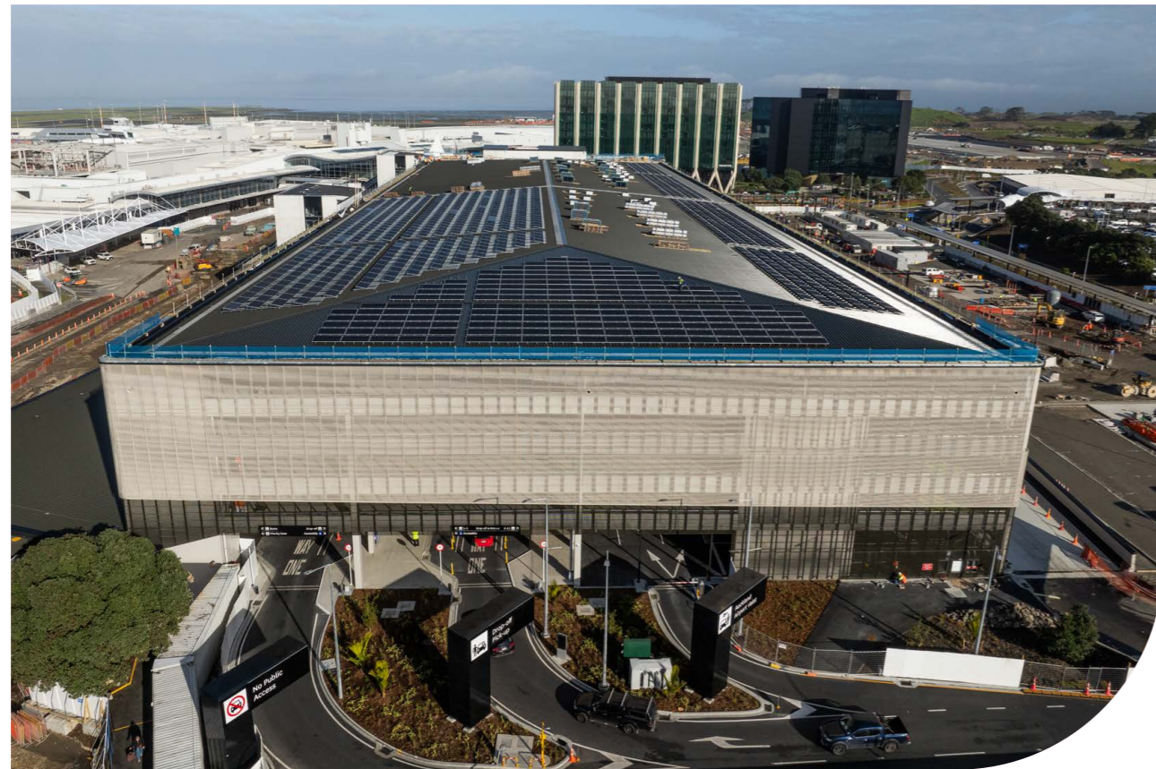
2 A 1.2-megawatt rooftop solar array installed on the roof of the Transport Hub.
