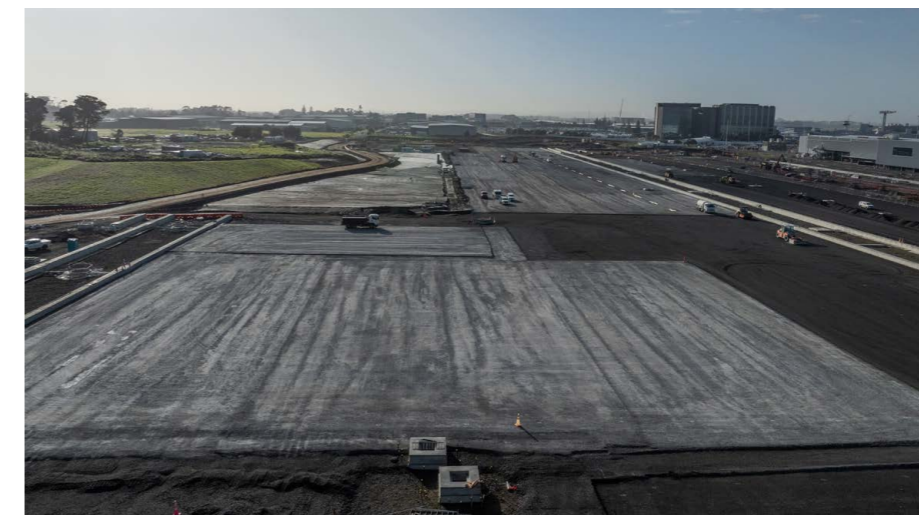
6 After extensive preparation, the airfield expansion was ready for paving to start in July 2024.
